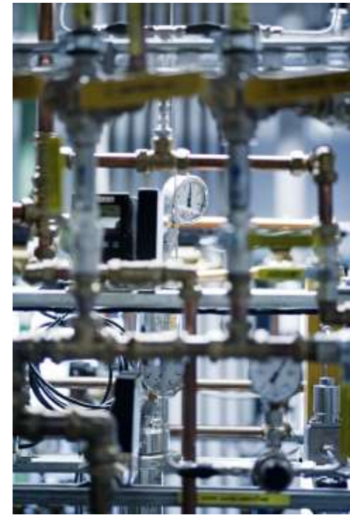
Gas mixing station Picture DGC
