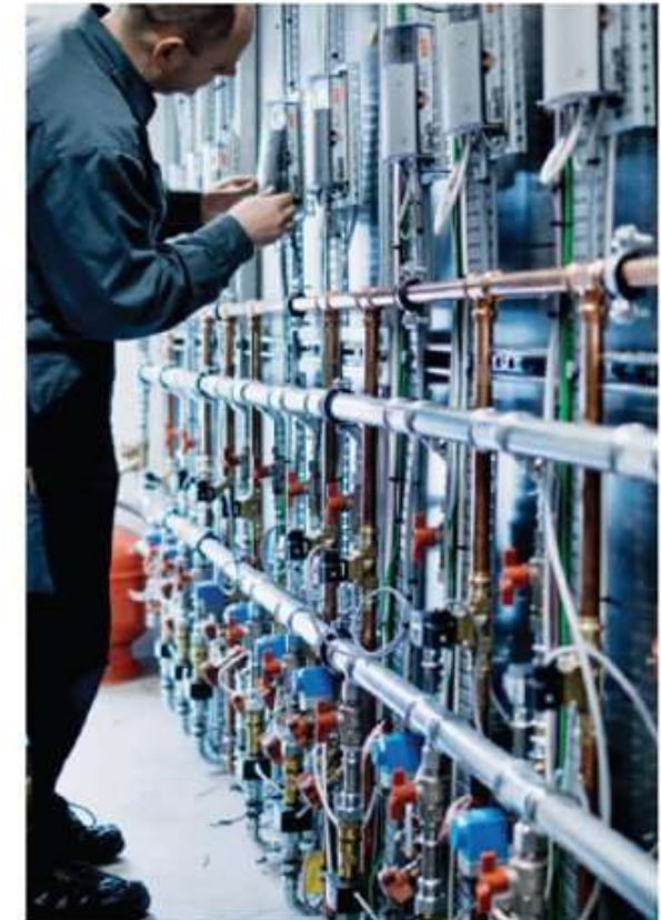
DGC's long term test rig is especially designed to monitor gas appliances performances over testing periods of several weeks or months.
