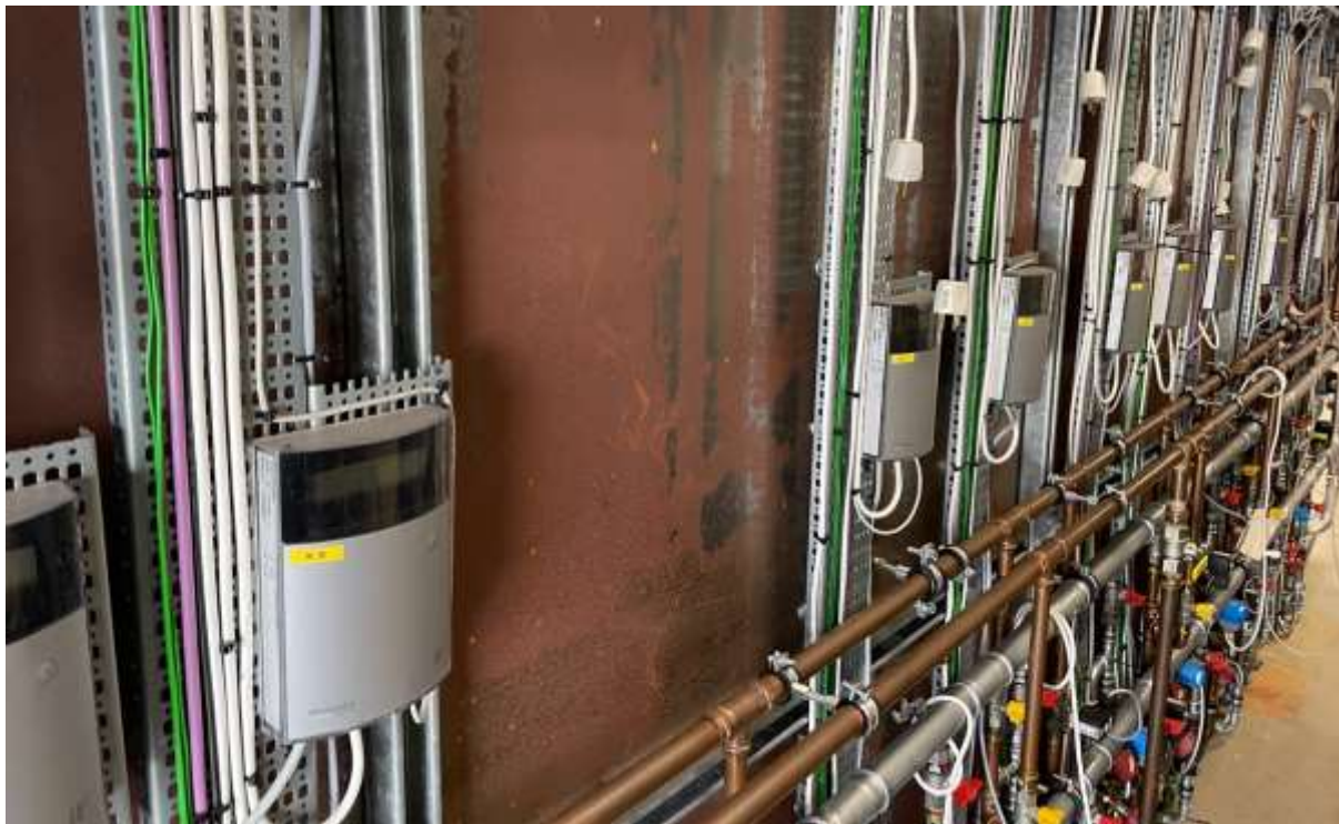
Figure 11: Outside the long test room, gas appliances water supply etc.
