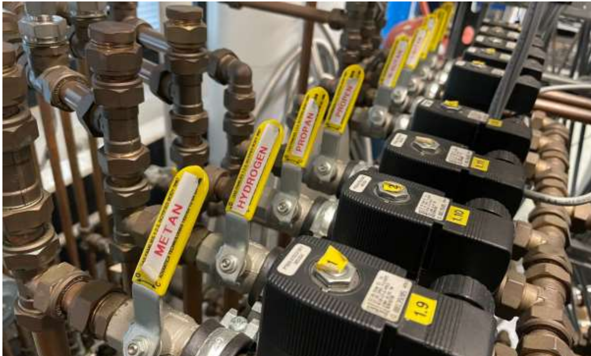
Figure 9: Details of the gas mixing station
