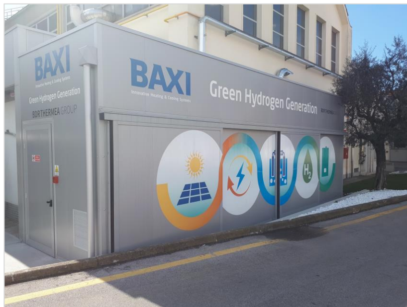
Electrolysers for Green Hydrogen (25 m 3 /h)
