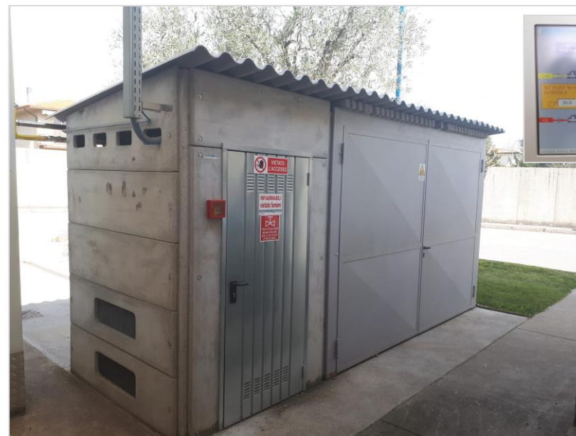
H 2 bottles Storage and mixing station
